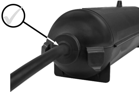
Picture 5: Cable entry correct
